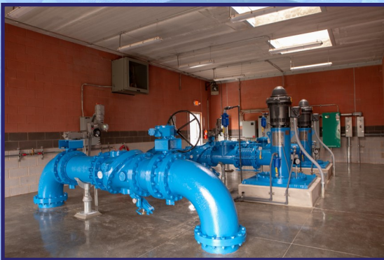
Hargrave Pump Station
