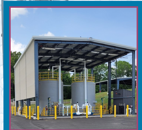
Bleach Bulk Tanks
